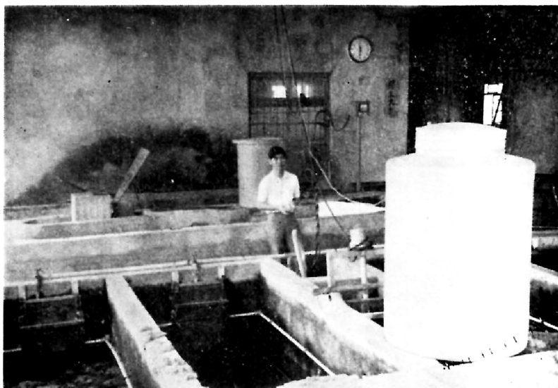
Fig. 7-4. The Immersion Tanks and the Automatic pH Control Equipment for Acid Treatment.
